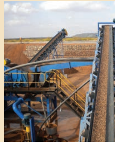
The plant at Diamcor Mining's Krone-Endora diamond project, in South Africa. Credit: Diamcor Mining
